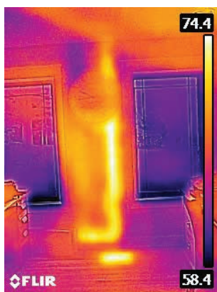
Warm Drain Pipe in Wall
