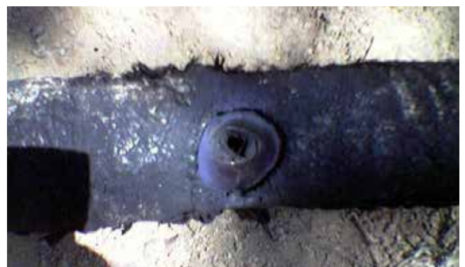
➤ Cable Fault in a 132 kV PILC cable
