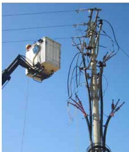
➤ connection to pole mounted cable terminations
