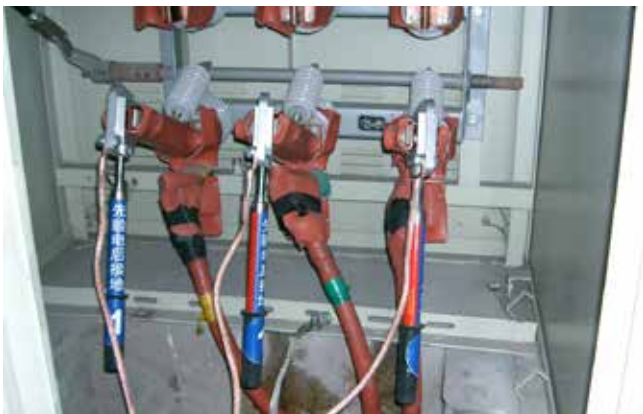
➤ Grounding of all phases
