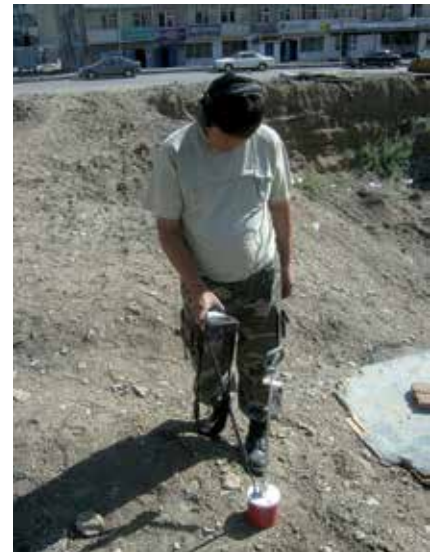
➤ field application acoustic fault location
